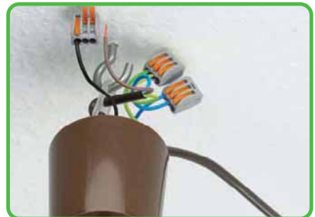
Lighting fixture connected with flexible power feed.
