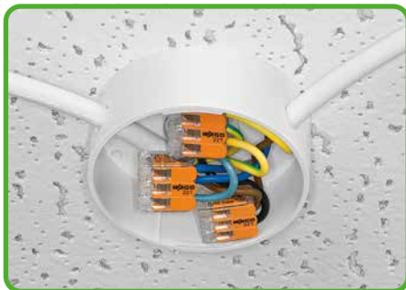
Lighting distribution in ceiling canopy
